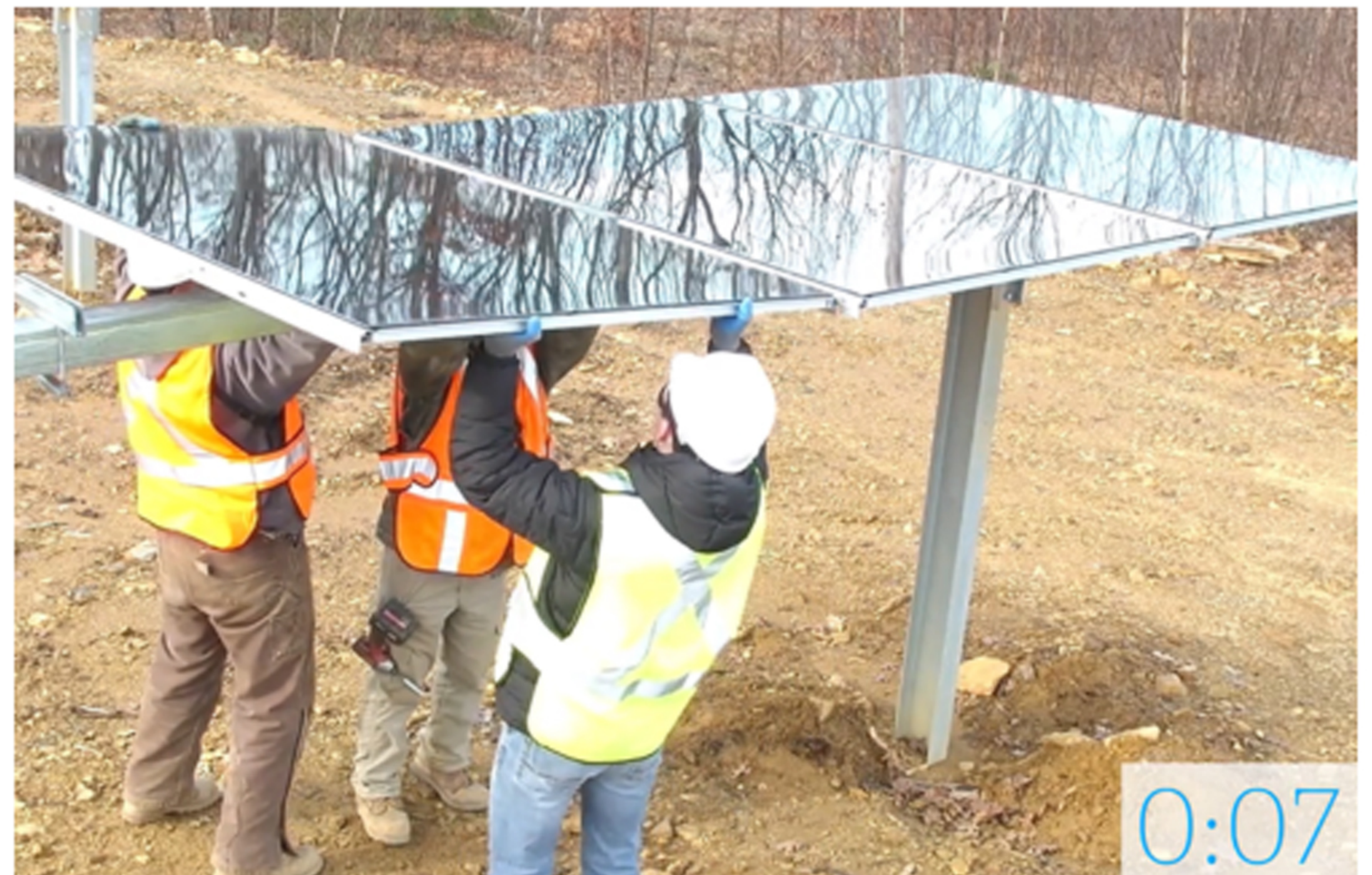
A crew of three was able to install a single First Solar Series 6 module in 31 seconds using GameChange Solar's SpeedClamp. Game Change Solar
