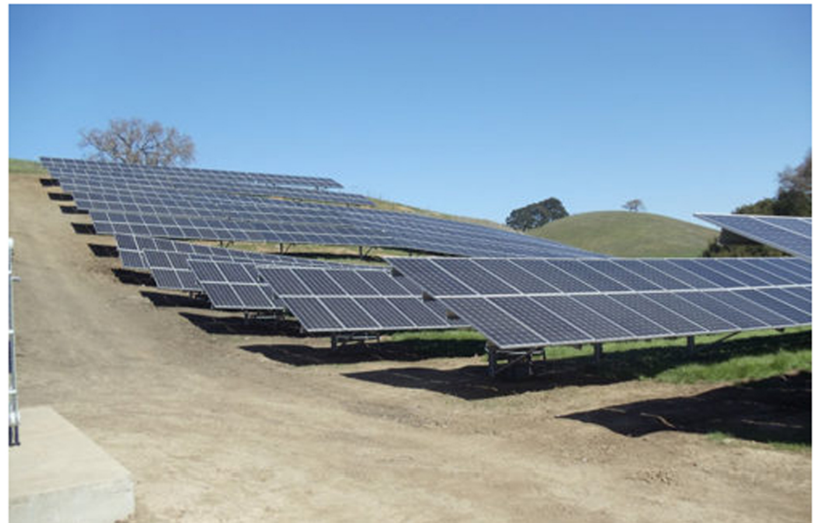
A ground-mounted solar array ascends up a hill. While it's simpler to install solar on flatter terrain, hills and undulating ground are feasible solar sites. RBI Solar
