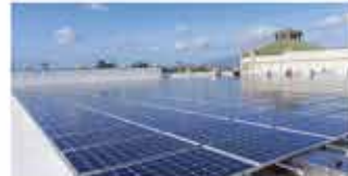
An array installer at a multi-building project for the U.S. Army at Fort Belvoir that used GC's Rapid Mounting System. Photo courtesy of GameChange Racking.
