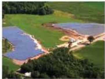
GameChange has secured backlog and pipeline for sales of nearly 1000MW in 2016. Image: GameChange Racking
